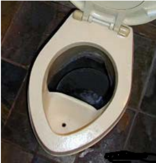
Urine Diversion Toilet
